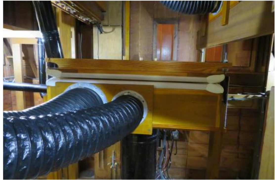
A view inside the organ chamber of the reinstalled Swell reservoir with new flexible wind hoses leading to the new outlet flange
